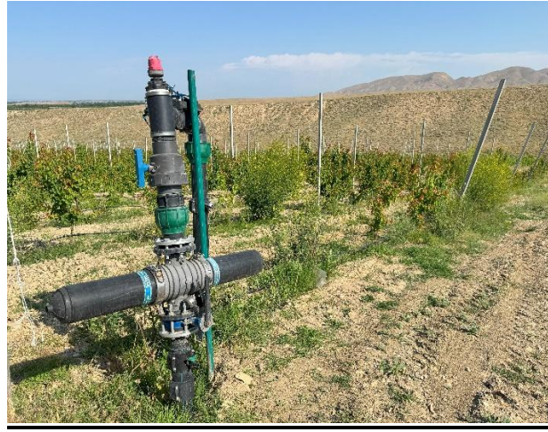
The head unit of drip irrigation system
