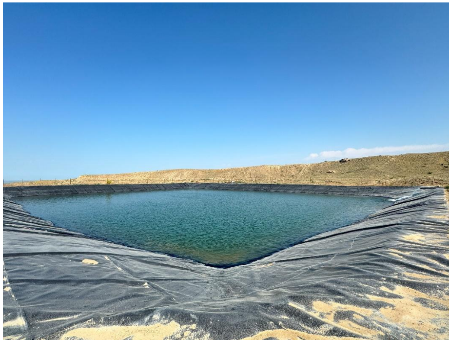
Geomembrane water reservoir for irrigation of orchards
